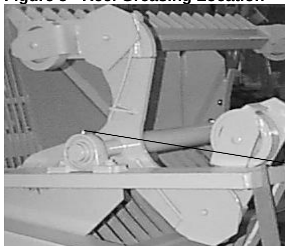
Figure 5 - Reel Greasing Location
