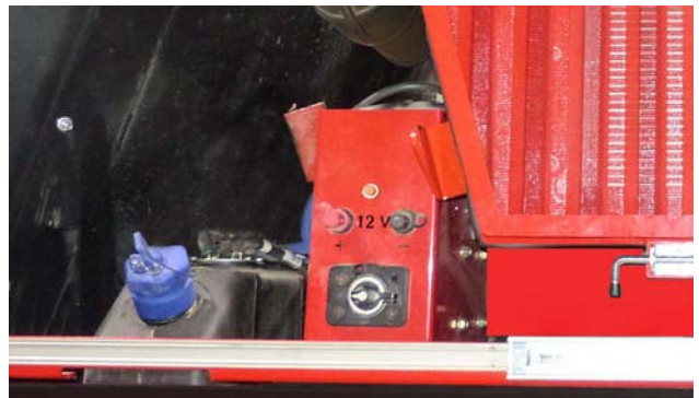
DEF Tank, Battery Shutoff
