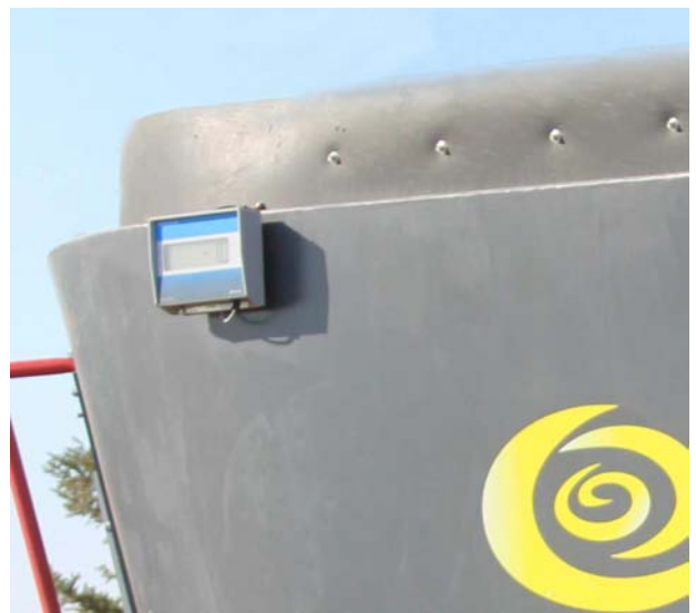
Remote Display Mounted on Tub Wall (Left Hand Mounting Shown)
