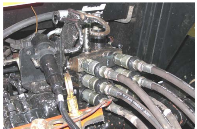
Inspect Hydraulic Hoses
