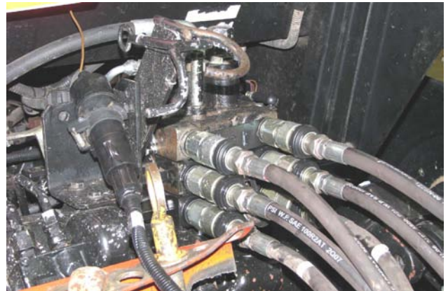
Inspect Hydraulic Hoses
