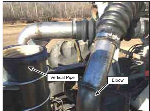
Figure 1.10 - Elbow Removed from Vertical Pipe
